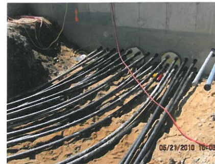
2 A loop of piping from each bore hole enters the building underground.
