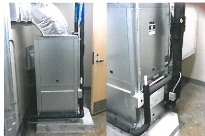
4 Heat pumps extract BTUs from the fluid and transfer it to air, which is blown through ducts into each room.
